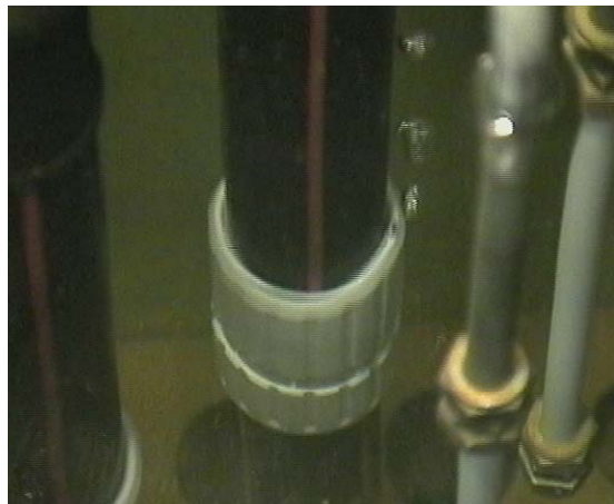
Figure 4 – Internal Pressure Testing – Leaking Coupler
